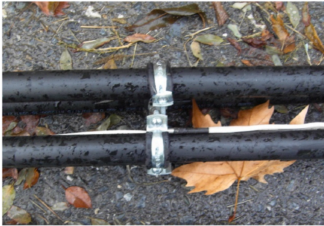
Fig. 3. Temperature sensor that located on pipe.
